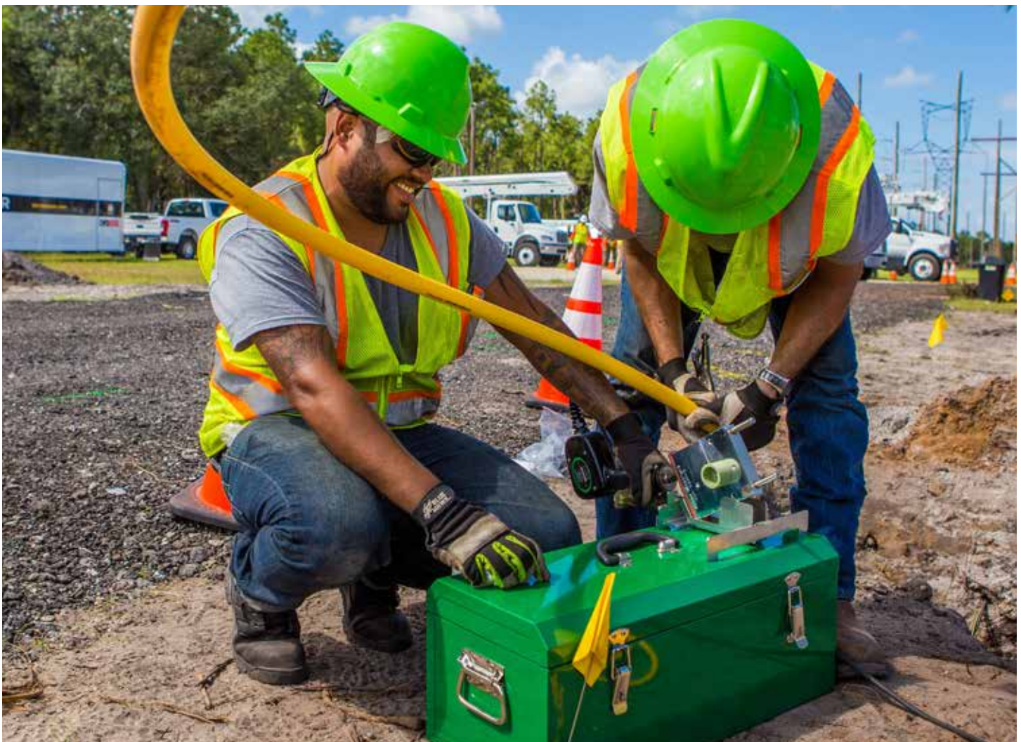
Students get hands-on training in the NLC Natural Gas Technician Program training yard, Florida campus.
