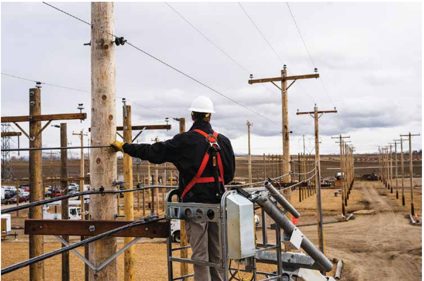
A portion of the NLC Idaho telecom training yard.
